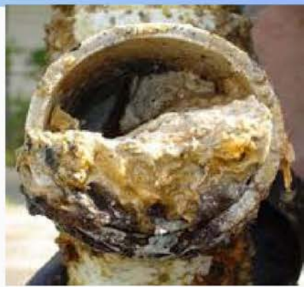
Picture of FOG in Pipes
